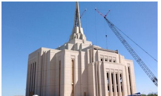
Temple of the Church of Jesus Christ of Latter -Day Saints (Gilbert, Arizona) Quik-Shield Spray Foam Insulation
